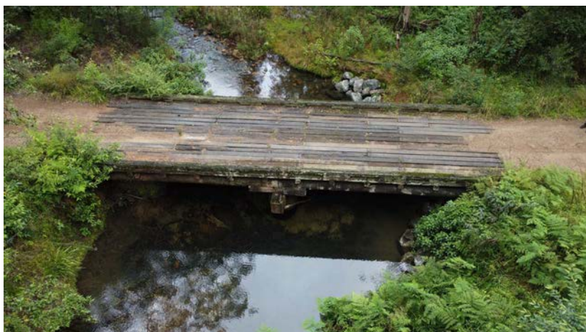
Floods significantly damaged this timber bridge on Blue Mountain Creek Road, Bulga. Image: Forestry Corporation
