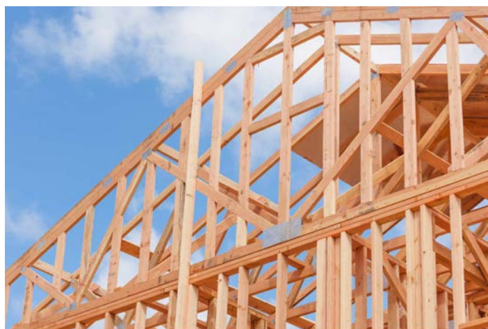
The Canadian Government is helping forest sector workers in Montreal and across the country to adopt the most cutting-edge technologies available to drive down costs and help the construction industry access the low-carbon Canadian wood products it needs to build more homes. Image: Shutterstock
