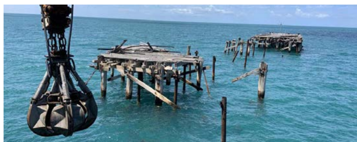
One Mile Jetty was badly damaged during Cyclone Seroj in 2021. A lack of jarrah means repairs are being made with imported merbau. Photo: Government of Western Australia Department of Transport
