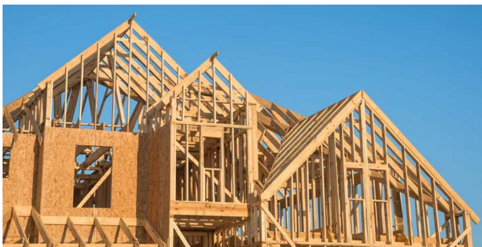
The project focuses on making it easier for builders, designers and engineers to work with lightweight timber framing, ultimately speeding up construction while using our forest resources more effectively.
