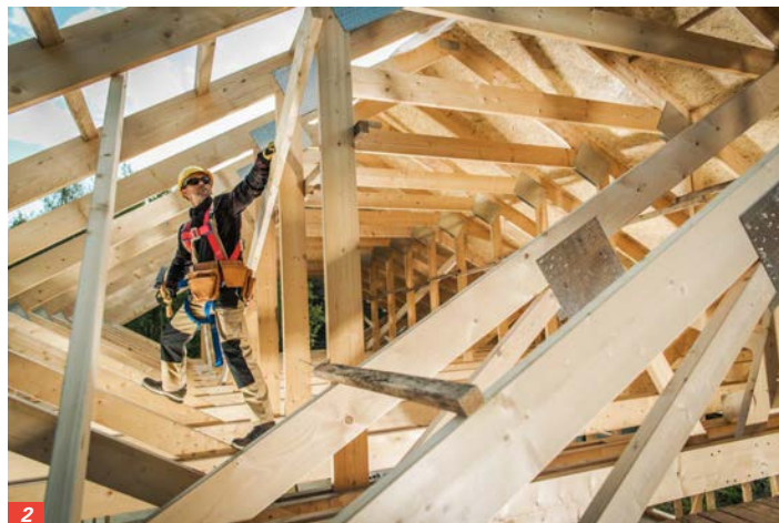
1/ Building sites already carry inherent risks. It is important to ensure that the culture helps to make sites safer not more dangerous.
