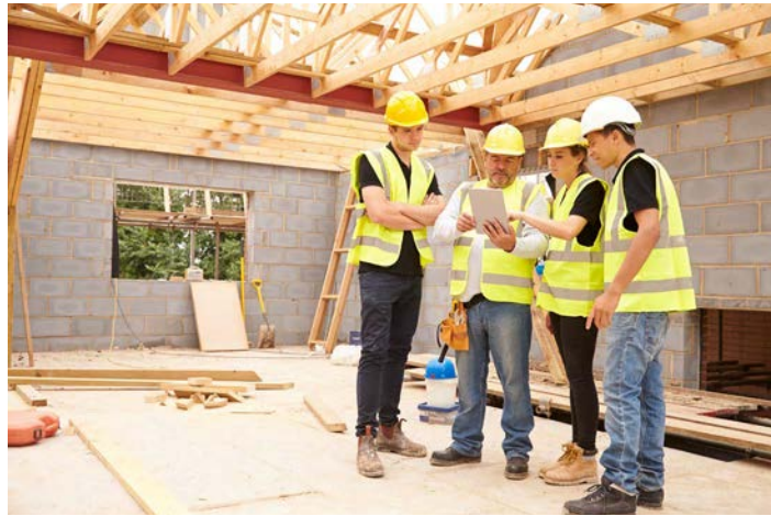
More apprentices are needed in construction and HIA has called for assistance to make them more affordable, as well as safer and more inclusive worksites. Image: Shutterstock/Monkey Business
